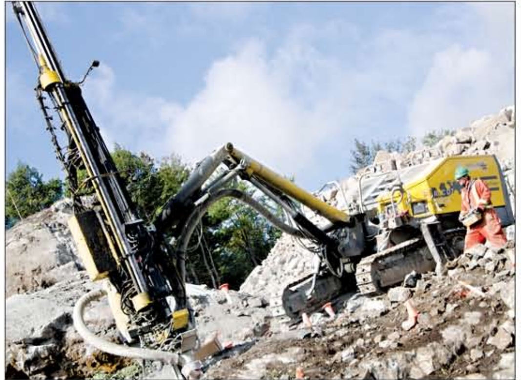
A Hwy 5 labourer with Couillard Construction drills some dynamite holes in a rock ridge across from Morrison's Quarry in Chelsea. The entire hill, along with several other large rock outcrops, will be completely blown up to make way for the highway extension to Wakefield. See pages 14-15 for a complete lowdown on what is happening to our Hills. Trevor Greenway photo
